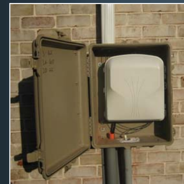
Wall mounted Peli 1600 case with telecommunications gear.
